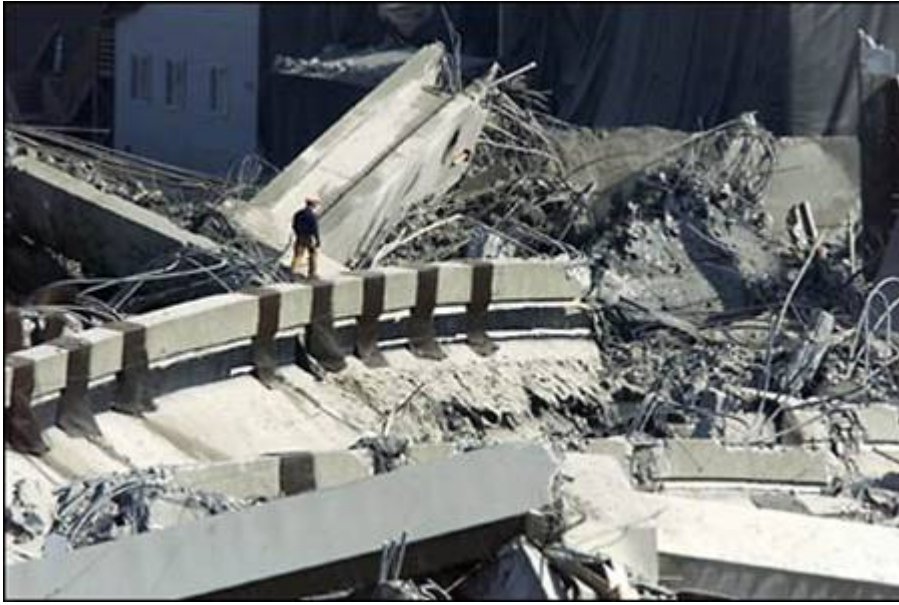
A worker strides across one of the Dome's fallen "ribs" after the implosion. (March 26, 2000)
