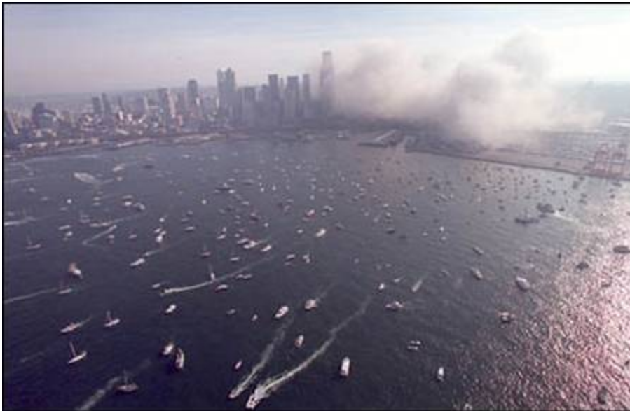
Boats packed Elliott Bay Sunday morning to watch the implosion from the water. Although Washington State Ferries attempted to stick to a normal schedule despite the demolition work, vessels were delayed by the marine traffic jam. (March 26, 2000)
